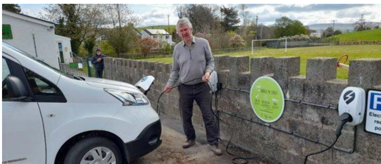
Charge My Street chargepoint at Thwaites Village Hall. Photo credit: www.nwemail.co.uk
