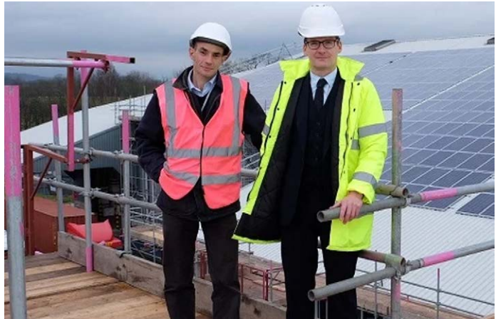
Directors Mark Cropper and Phil Davies at Burnside Community Energy Ltd on the roof of James Cropper plc. Photo credit: BCE
